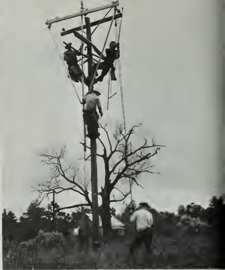
A Santee crew, working while the lines are hot, installs a new cross arm on a pole.
